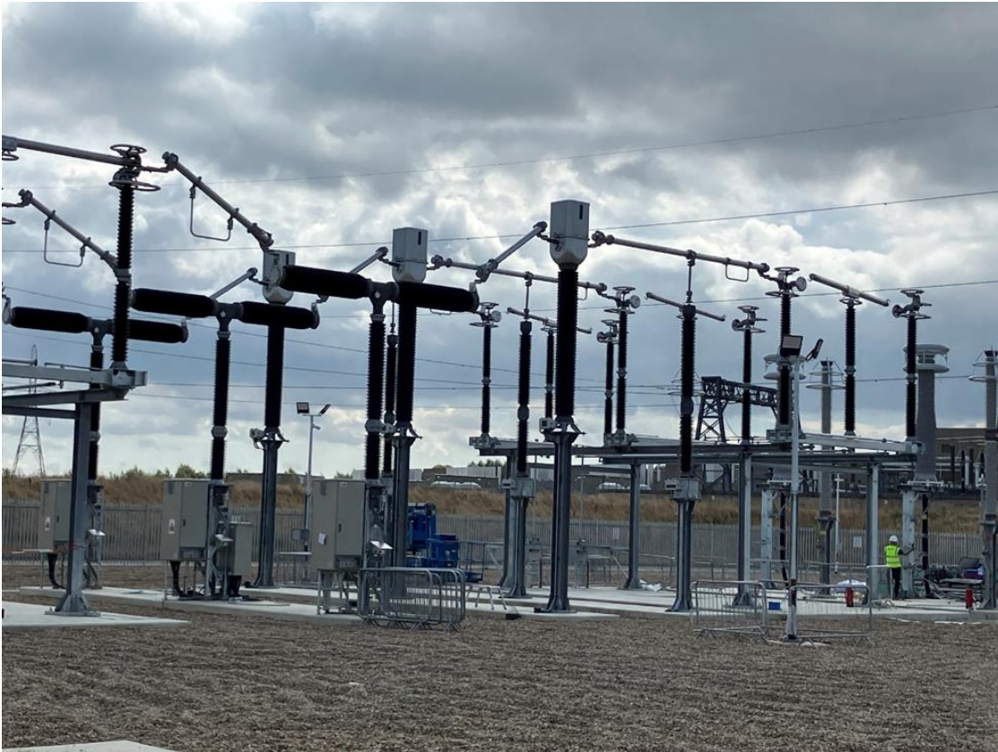
Plate 5-5 Typical 275 kV substation equipment
